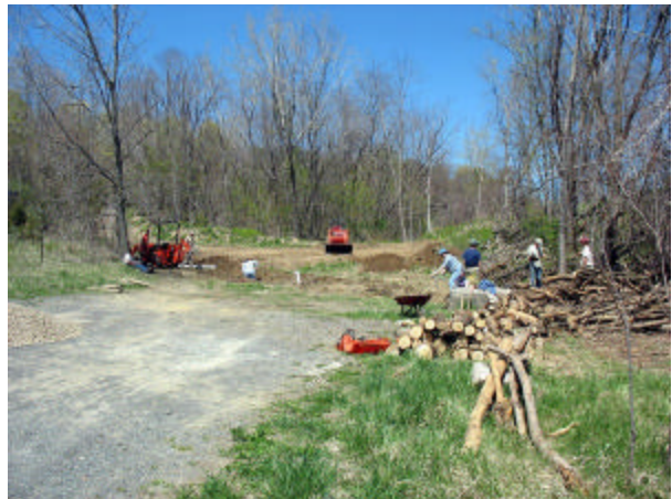
Volunteers working on the parking lot at Clarksville, picture by Mike Chu
